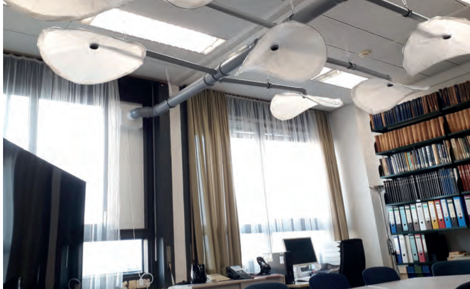
Fig. 2: Installed ventilation system with extractor hoods.
